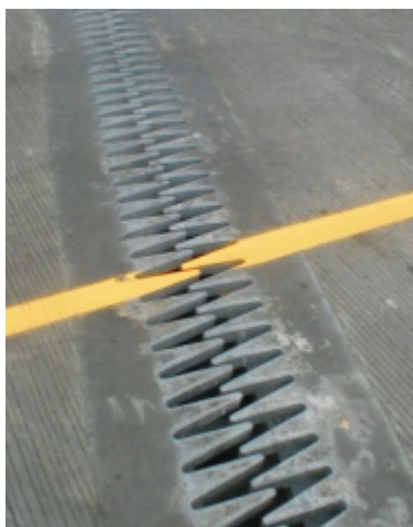
Figure 6.1: Thermal expansion joints in a roadway.
